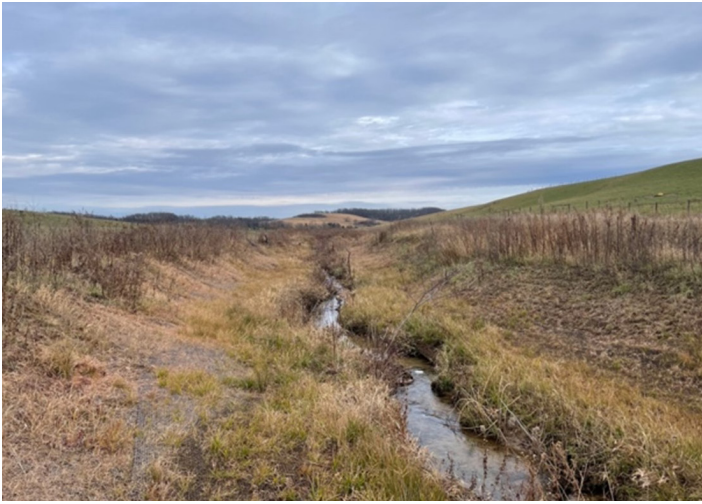
Figure 6. Vegetation growth six months (12/15/2021) after coir mesh installation along Ruby Run, Preston County, West Virginia, USA.
