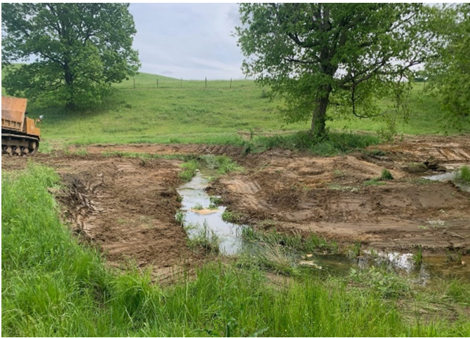
Figure 2. The streambank grading of Ruby Run and the adjacent wetlands, Preston County, West Virginia, USA. (Note: All photos taken by Andrew MacKenzie)
