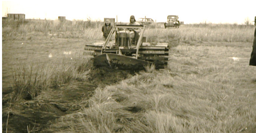
FIGURE 9. Scavel plow clearing debris from a mosquito control ditch circa 1940-1950s. Mechanized ditching patterns are ubiquitous from Massachusetts southward, often overlay previous agricultural ditching patterns, may not adhere to tideshed boundaries or original marsh slope, and develop highly compacted embankments on both sides of ditches. (Photo credit CT DEEP.)
