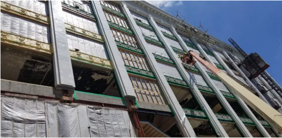
GFRP Replacement Spandrels
