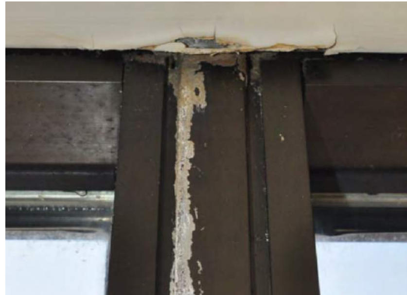
Water Infiltration at Windows
