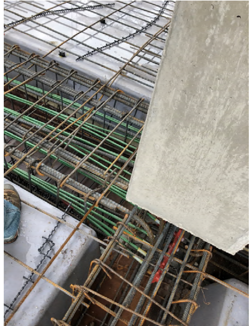
General bar congestion and concrete elements
