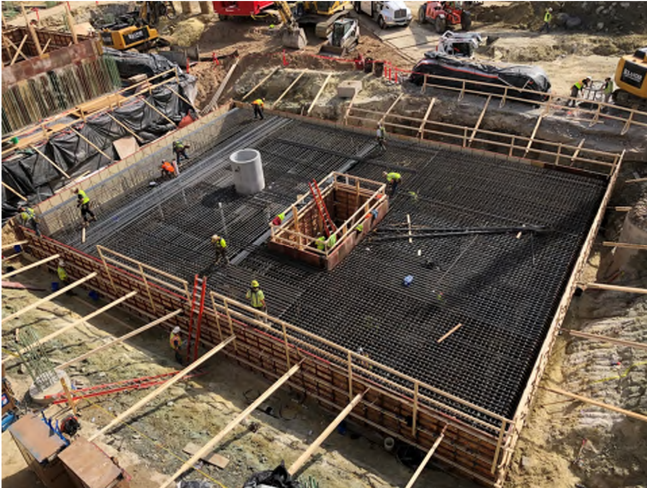
MAT AT SHEAR WALL CORE 2 LAYERS GR75 #11@6" AT BOTTOM AND GR75 #11@6" TOP
